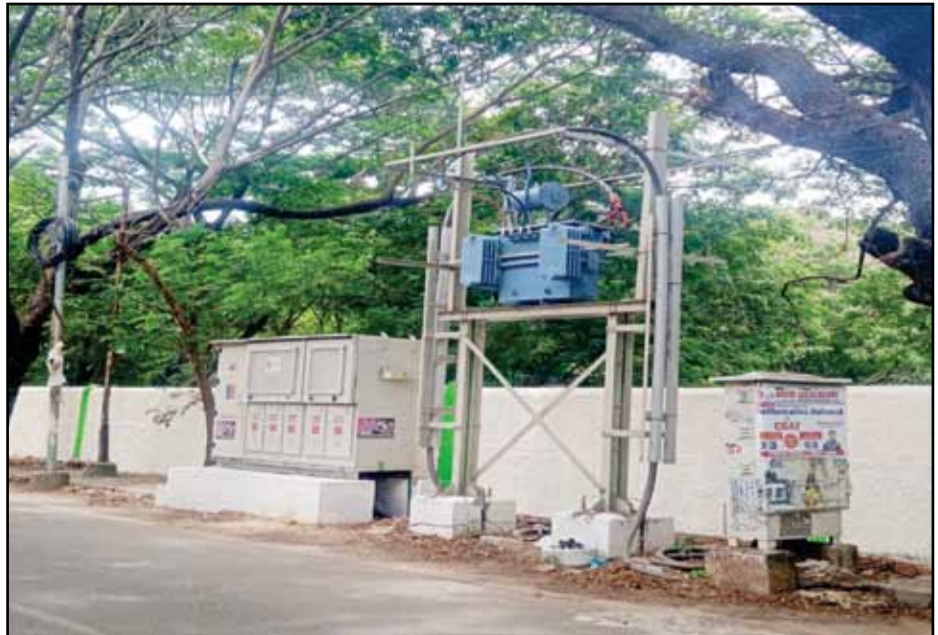
The Electricity board officials erected a new transformer in x block. The x block people's and pedestrians happy to see that .
